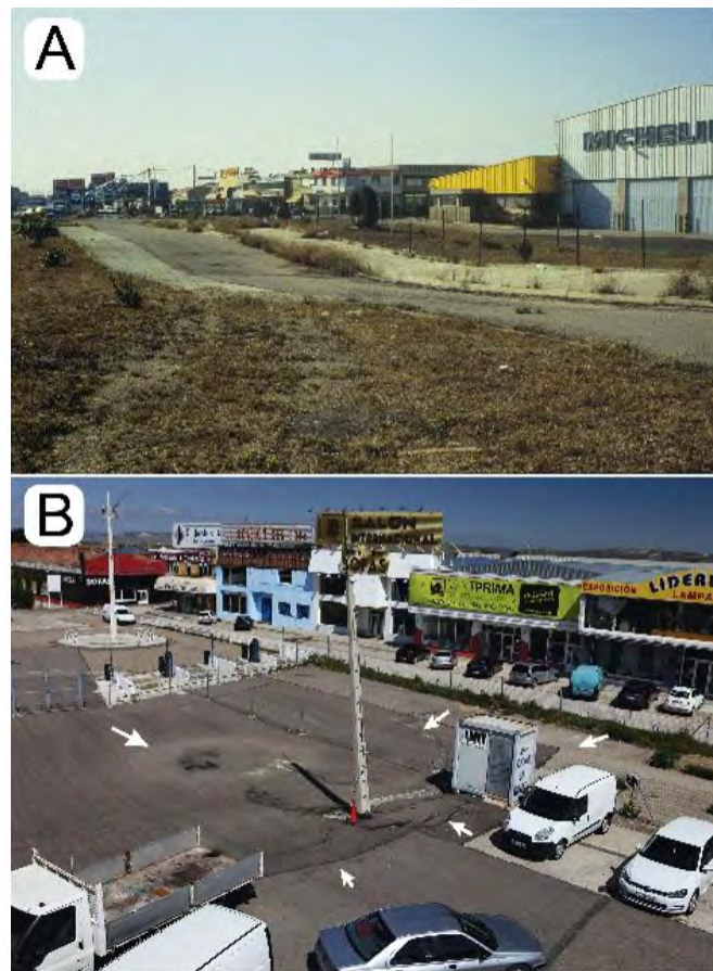
Figure 5. Images of the Logroño highway sinkholes. (A) Photograph taken on June 1996 at the NE sector of sinkhole 1 before the enlargement of the highway and the construction of the currently existing department store. Note the conspicuous sagging of the service road and the sidewalk. (B) Image of sinkhole 2 taken on April 2016 affecting a recently asphalted surface within a fenced area. The left arrow points to the deeper part of sinkhole and the arrows on the right mark the outermost cracks.
